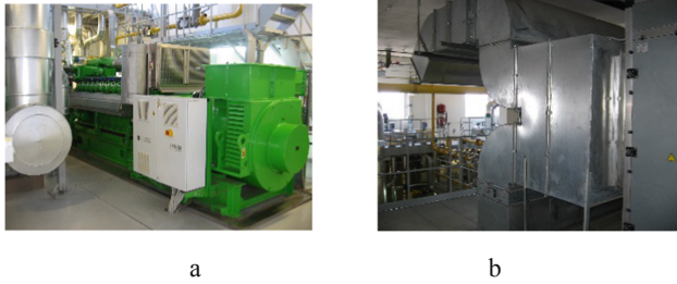
Fig. 1. Cogeneration gas engine module JMS GE Jenbacher (a) and waste heat recovery central conditioner for cooling engine room intake air (b)
